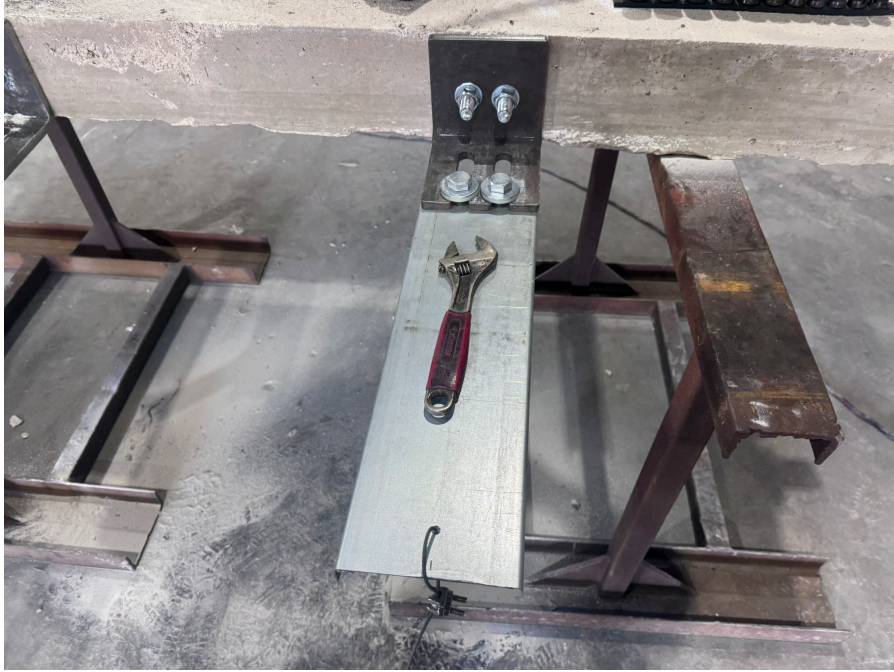
Photo No. 5 Dual Load Bearing Assembly
