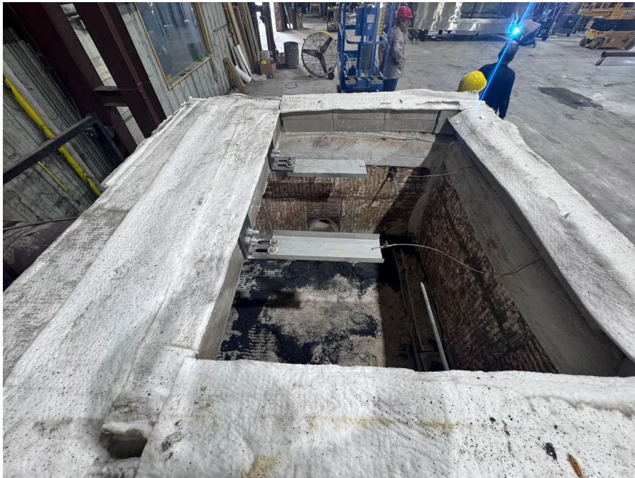
Photo No. 12 Connector Assemblies Placed into Furnace Prior to Test 2
