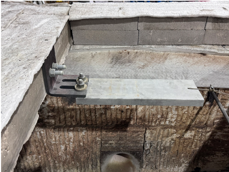
Photo No. 14 Dual Load Bearing Assembly
